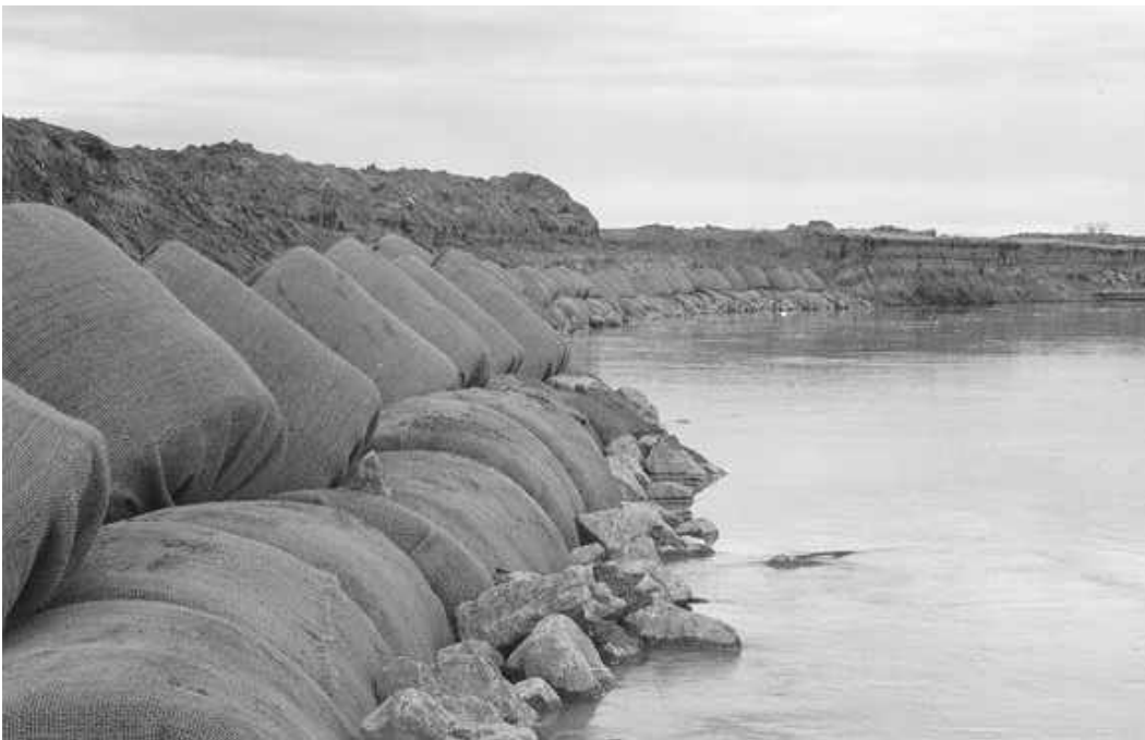
Figure 9. Photo of bioengineering project on upper Missouri River where large rock (1.5 Tons/lin ft) was used as toe protection below large coir-covered haybales, also forming part of the toe.
