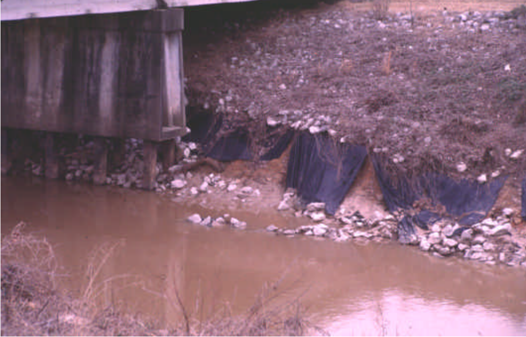
(c) Damage to Infrastructure
