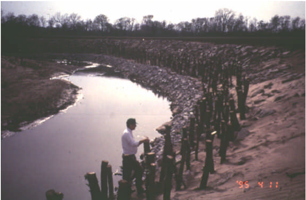
Figure 7.9 Longitudinal Peaked Stone Toe Protection In Combination With Willow Post Upper Bank Protection
