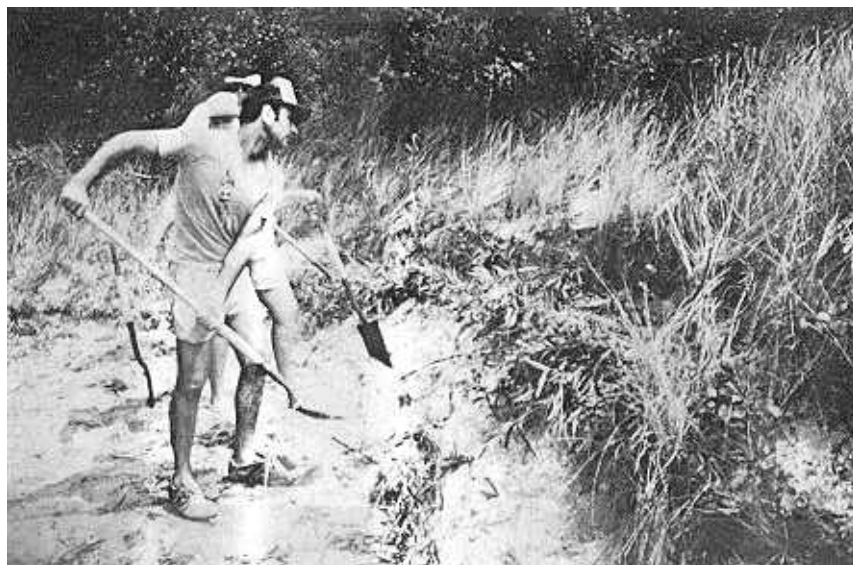
Figure 29. Installed section of brush layering. Note that brush has leaves because of a workshop setting. Normally, the brush would be without leaves because of installation during the dormant season.
