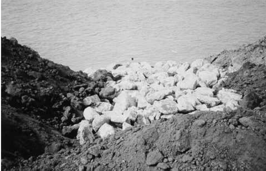
Figure 4. Rock refusal used on an upper Missouri River bioengineering project. Note that it is keyed back into the bank to prevent flanking of the upper and lower end sections of the project.
