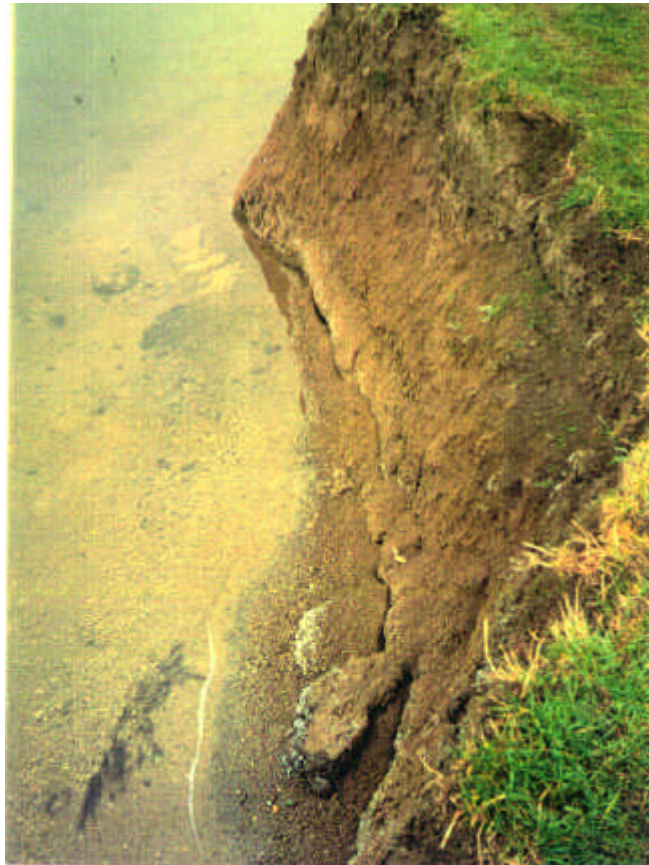
Figure 2.22 Erosion Generated by Freeze/Thaw
