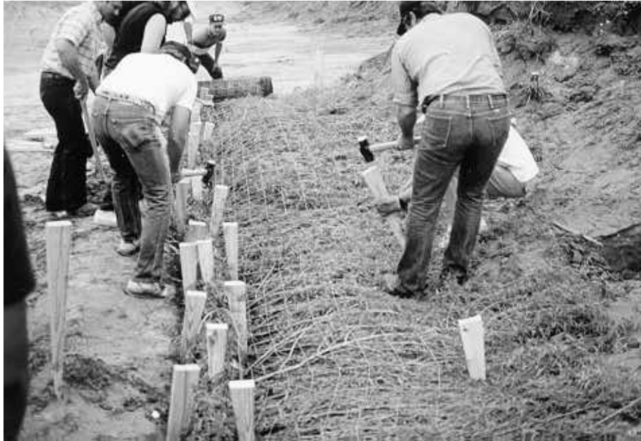
Figure 27c. Stretching the woven wire tight and securing by wedge-shaped stakes. Also, the wattling bundles are then laid over the top of the basal ends of the willow in the trench and secured tightly with wedge-shaped stakes.
