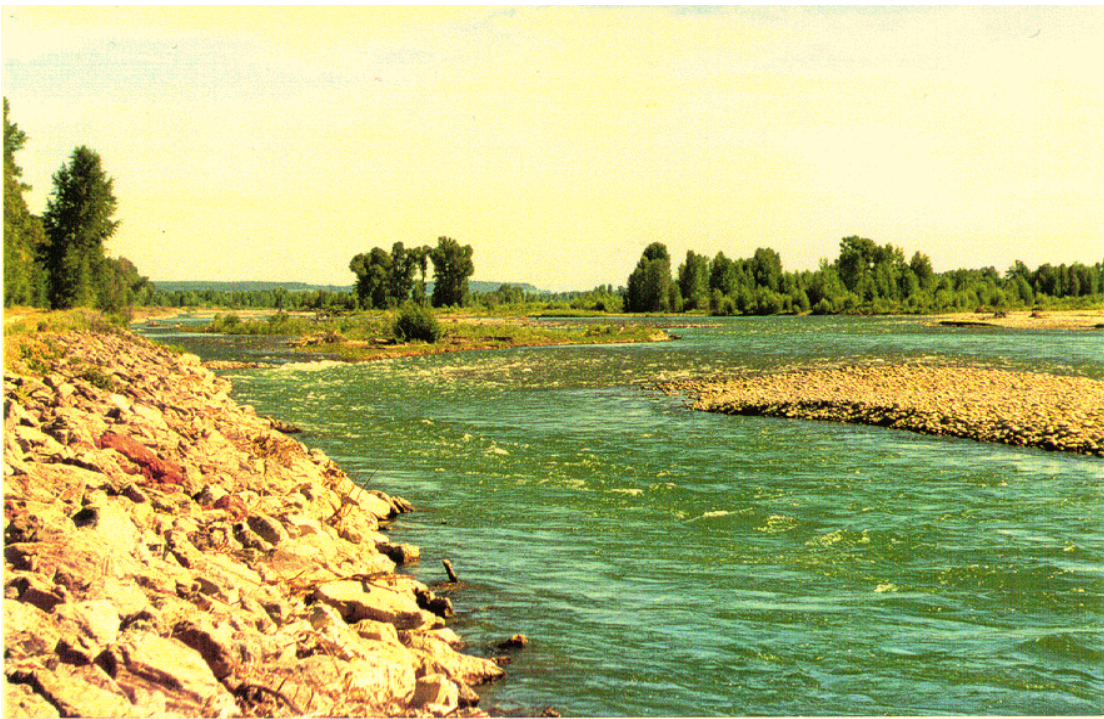
Figure 2.20 Erosion Generated by Impinging Flow
