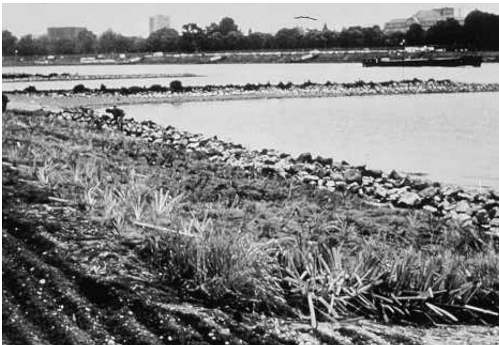
Figure 12. System of bioengineering treatments such as geotextile coir mats with planted vegetation on them placed above a rock roll toe and between large rock transverse dikes.
