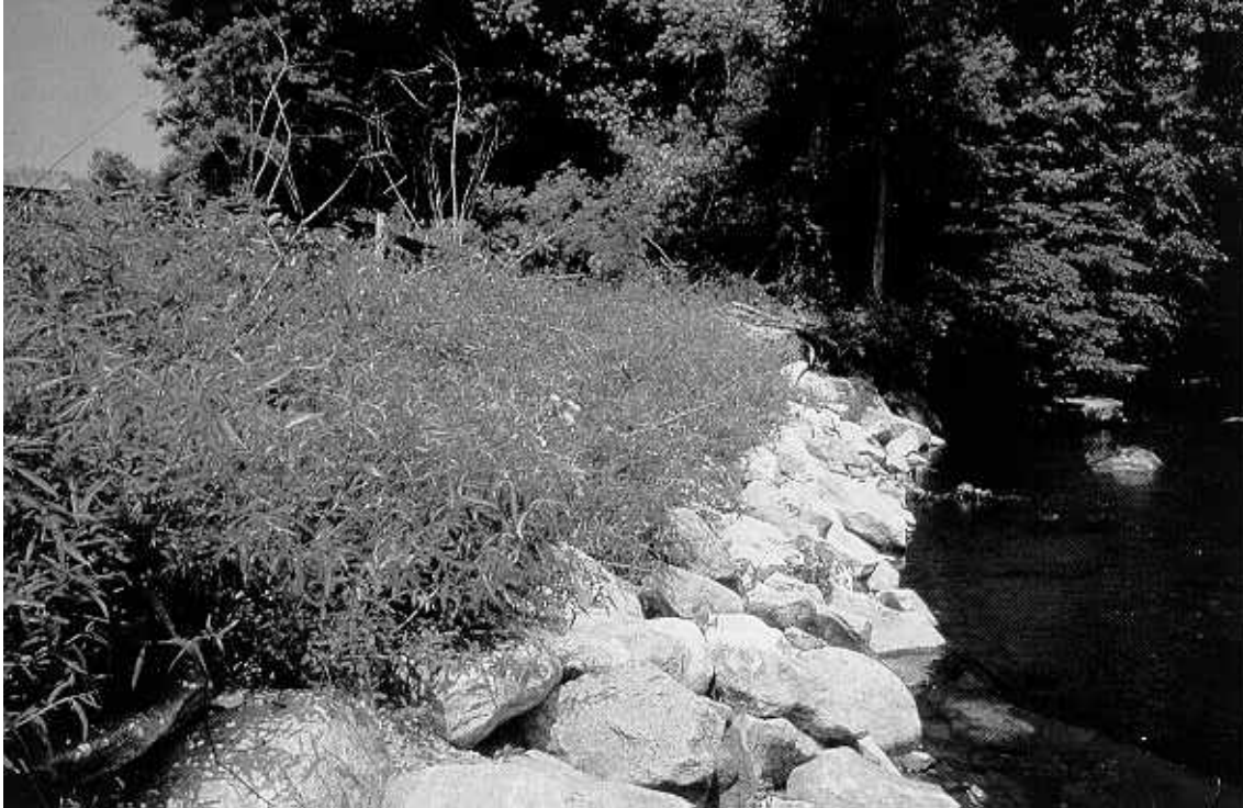
Figure 30. Brush layering with willow and dogwood branches after one growing season; installed above a rock toe (to prevent undercutting) on the Little Patuxent River, Maryland. (From Bowers, 1992)
