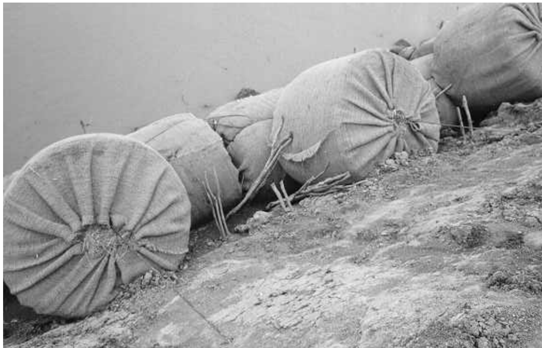
Figure 10. Vegetation in the form of dormant willow posts (discussed later) was placed landward of the rock and haybale toe.
