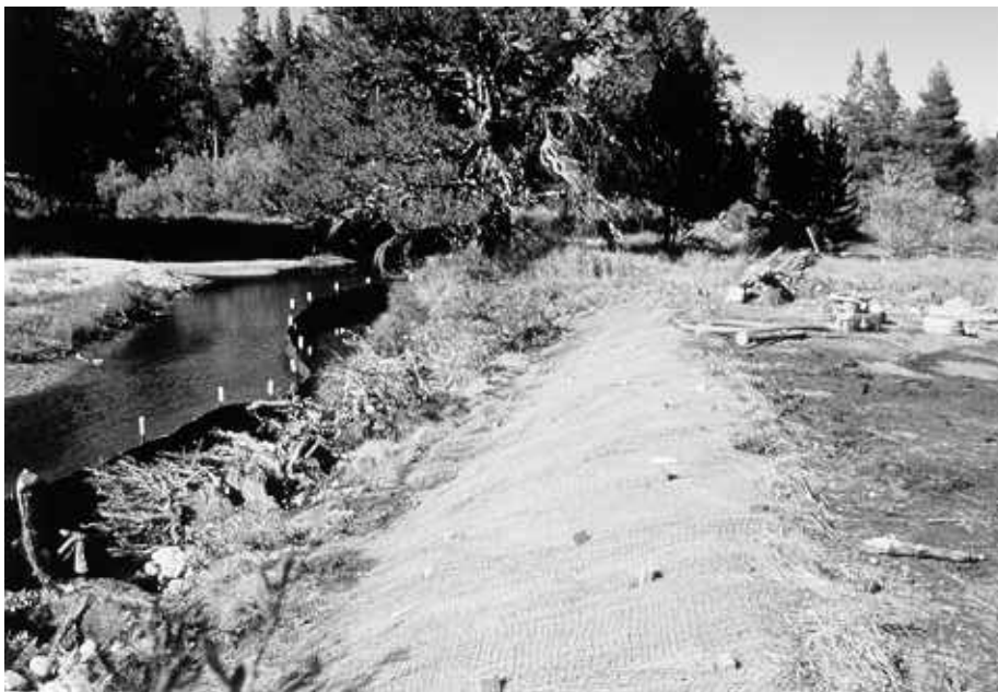
Figure 38. Burlap and coir woven fabric laid over sedge and grass seed, Upper Truckee River, California. Note that the fabrics were keyed in at the top and bottom in trenches and securely staked with wedge-shaped stakes. (Photo courtesy of Interfluve, Inc.)
