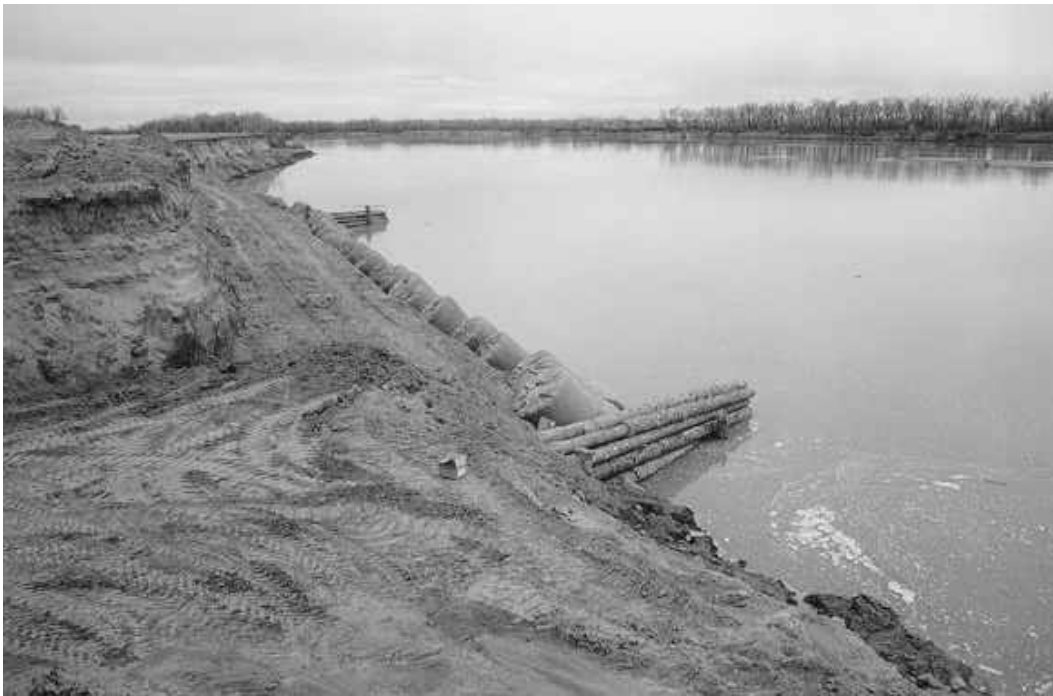
Figure 3. Timber cribs serving as deflection structures on the upper Missouri River to direct current away from the bank where there are bioengineering treatments.
