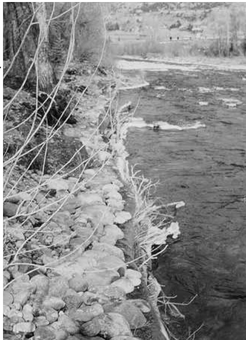
Figure 18. Installed log revetment with coir geotextile roll combination, Roaring Fork River, Colorado. Wetland vegetation is seeded or planted in backfilled soil placed in a depression between the revetment and the land. Rock is placed on top to prevent scour.
