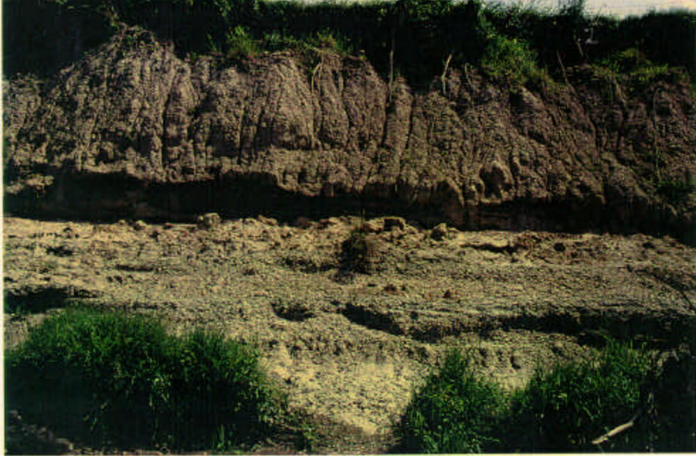
Figure 2.21 Erosion Generated by Piping
