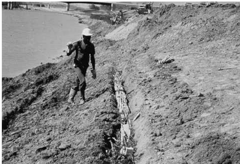
Figure 39c. Wattling (fascine) bundle being installed in the bank zone. Note that wattling should not be covered completely with soil; leave top 2-3" exposed for sprouting purposes. (Photo courtesy of Ms. Robin Sotir, Robin Sotir & Associates)
