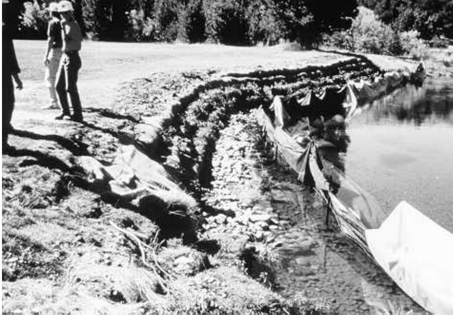
Figure 32. Vegetative geogrid during construction on the Upper Truckee River, California, near South Lake Tahoe. Note rock toe that was keyed into channel bed and bank to prevent undercutting. Photo was taken in October 1993.
