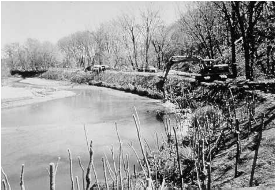
Figure 34. Dormant willow posts, coir geotextile roll, and cedar trees being installed at Court Creek, Illinois, April 1993. (Photo courtesy of Mr. Donald Roseboom, Illinois State Water Survey)
