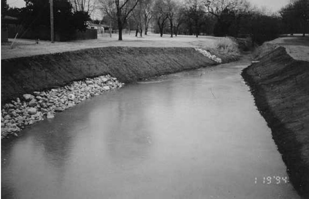
Figure 8. Photo of weighted rock toe revetment extending up the bank. It extends about 1/3 the distance up the bank. This photo shows the stream above low-flow conditions.
