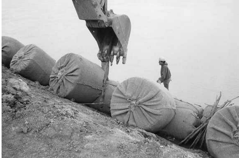
Figure 36. Use of “The Stinger” to create pilot holes for dormant willow posts on the upper Missouri River (CE project, Omaha District).
