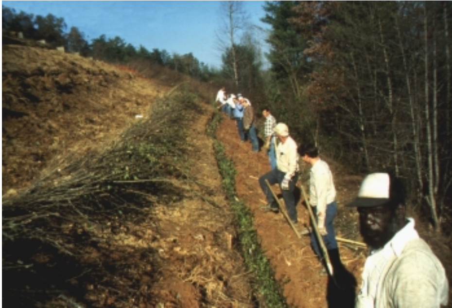
Figure 18-8a During installation (note size and depth of trench to size of live fascine bundle)
