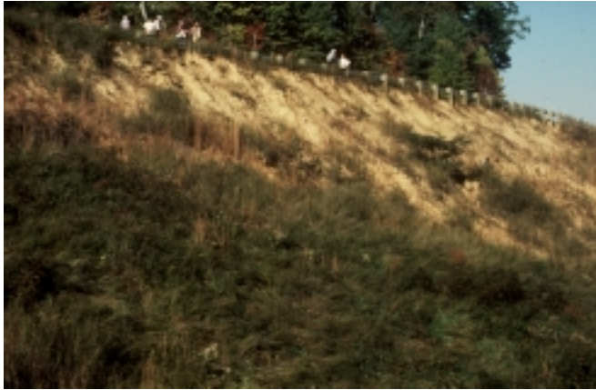
Figure 18-1a Eroding fill slope
