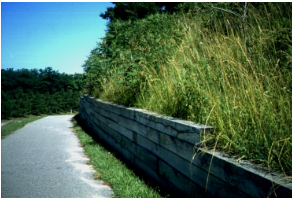
Figure 18-26 Low wall at the base of a slope with vegetation on face of slope (Donald H. Gray photo)
