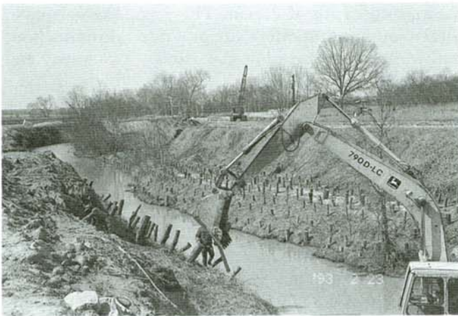
Figure 3. Planting Dormant Willow Posts With Hydraulic Hoe and Ram at Site V3.
