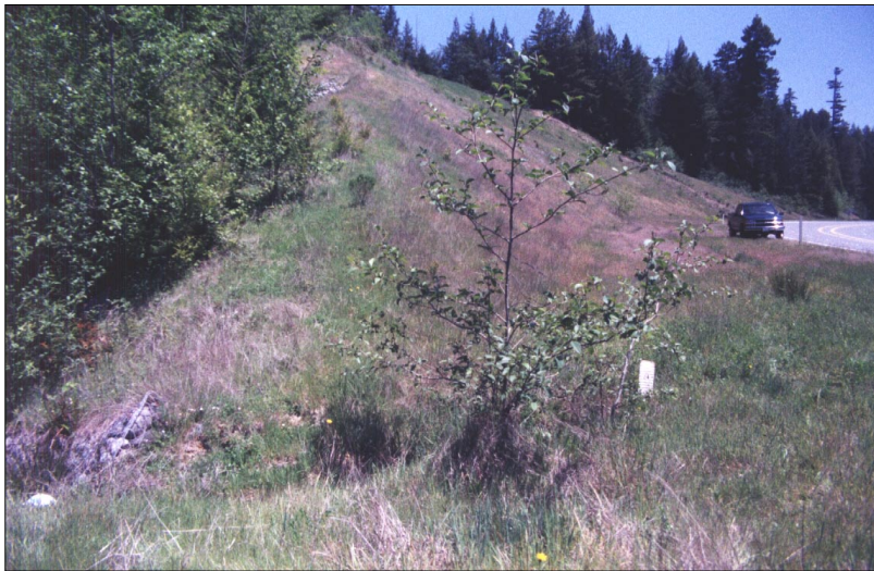
Photo 57. Where 18" deep gully from slope and shoulder runoff connects to gabion channel (at left). Top 1-foot of 30" white scale in gully is visible. Super-elevated road drains away from gully toward right.
