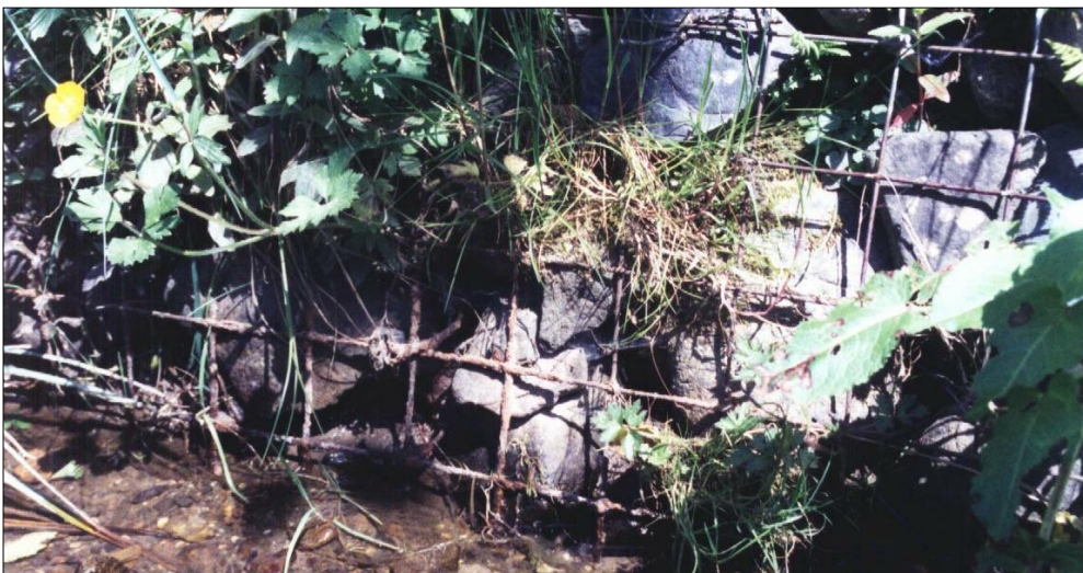
Photo 42. creek bed and wall under test panels, 26 May 1999. most bedload and high-velocity suspended sediment did not get here. Rust on low wires, no rust above ordinary high water, 1-foot above creek bed.
