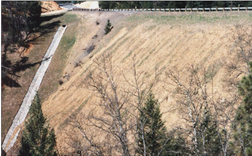
Photo 120. March 1988, gabion downdrain trapped sediment during 1 st wet season. Sediment from eroded embankment (right) 15H:1V, gabion downdrain slope is 2H:1V.
