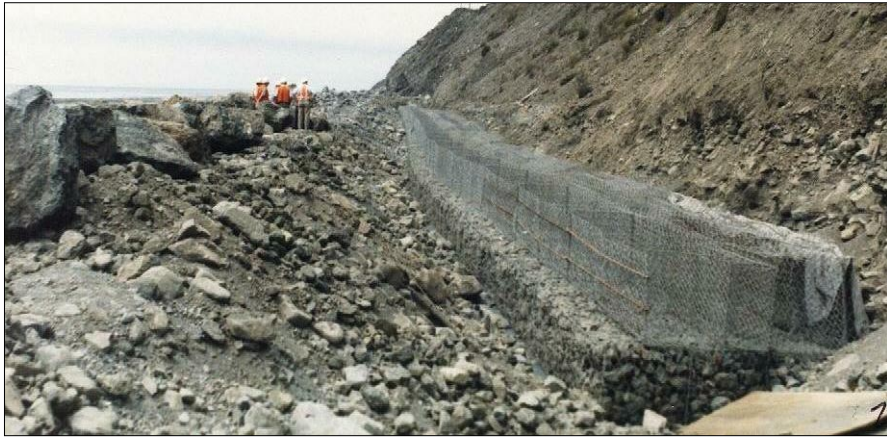
Photo 89. Building north wall with PVC-coated gabions, product 5, on 7 Aug 1985, looking northerly, near post mile 8.1. Base tier completed of 7-tiered, step-faced wall, bottom gabions at about elevation 4 feet.
