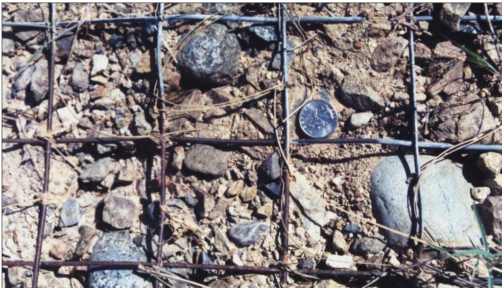
Photo 124. Rusted wire at edge of splash zone (downhill at top of photo), after 12 wet seasons, 28 May 1999. Zinc (dull gray, likely zinc carbonate) still present (by shiny quarter) indicates relatively little abrasion. Rusted wire diameters not significantly different than wires with zinc.
