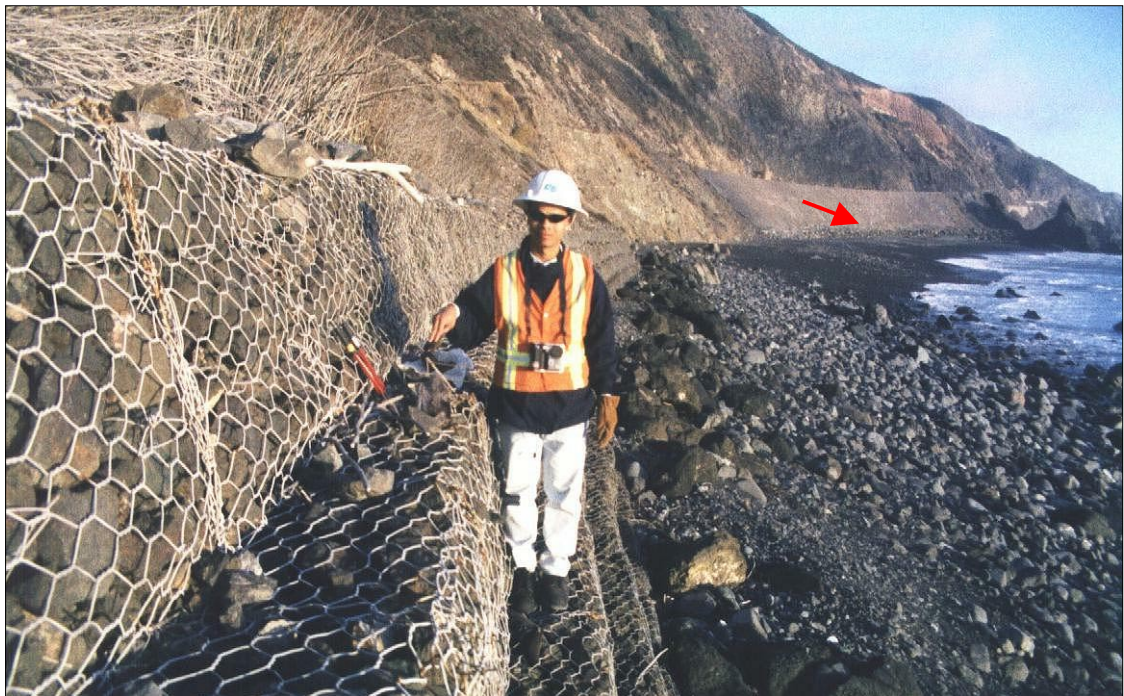
Photo 98. Observer points-out where sloughed rocks severed some gabion wires, gabion rock-fill is still contained. North RSP (arrow) is about ¼ mile distant. Both walls are OK after 16 wet seasons (assessed by maintenance, May 2001), despite broken wires from rock impacts.
