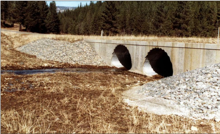
Photo 63. Inlet of double 10'-11" wide x 7'-1" high structural steel plate arch culverts which convey Mohawk Creek under route 89. Flow is continual in normal water-years. Culverts and gabion mattress slope protection, 1½ years after construction, 6 Feb 1991. At toes of slopes, gabion counterforts (3' x 3' cross section) were concreted during construction. Toe at creek has 27-foot plan view radius (left, far side) and 40-foot radius (right, near side). Counterforts built 3-feet below culvert invert elevation for possible local scour.
