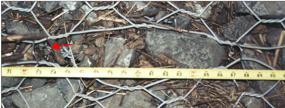
Photo 142. Second of 3 out-of specification joints, near 73-inch mark (arrow), fastener is not interlocked, then toward right, 2 fasteners are missing. Joint near high water, submerged by January 1997 flow, as indicated by drift (floating vegetative debris left behind after flood stage drops).
