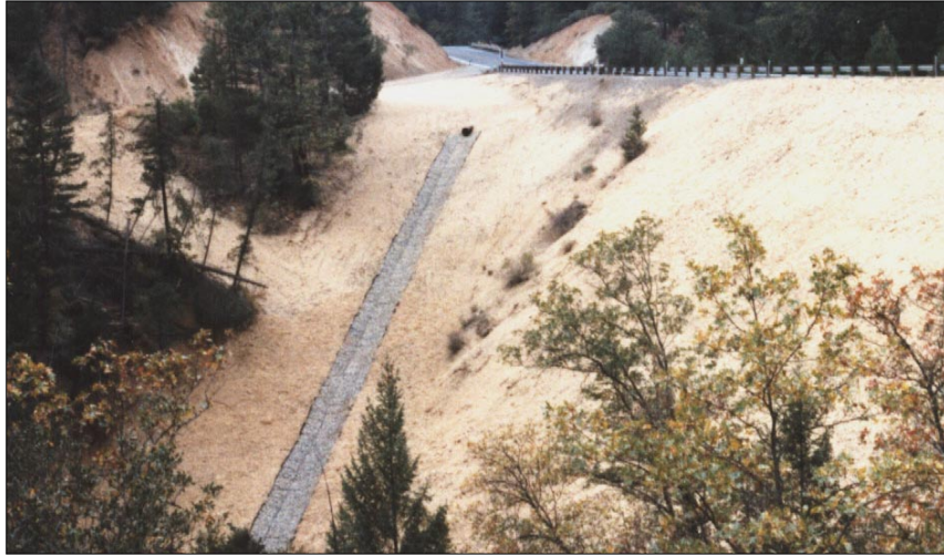
Photo 119. Completed gabion downdrain and slopes, Oct 1987. Road cut (top center of image) part of relatively small drainage area (less than 5 acres) that drains to culvert at top of downdrain.
