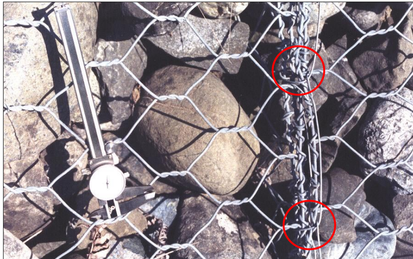
Photo 55. At this and other sites, we measured wire diameters of full-scale gabion facilities and inspected job quality. Several joints were partly "out-of-spec". Caltrans requires alternating single and double half-hitches at 4-inch nominal spacing, circled ties are single half hitches at 6-inch nominal spacing. A feature "within spec" is that all wires of the joint were enclosed by standard tie wire in a single pass. 26 May 1999
