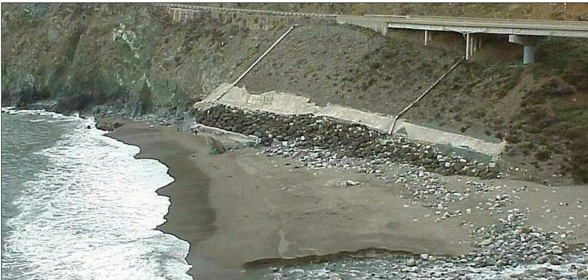
Photo 157. 8-ton rock buttress after 5 wet seasons, 14 Mar 2000, looking northeasterly. So far, rock is OK as scour countermeasure for toe of slope below abutment 10 and piers 9, 8, and 7 of bridge no. 44-0058.
