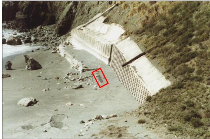
Photo 152. Partially exposed gabions (box), 10 Mar 1992, looking northerly. See photos 150 and 151.
