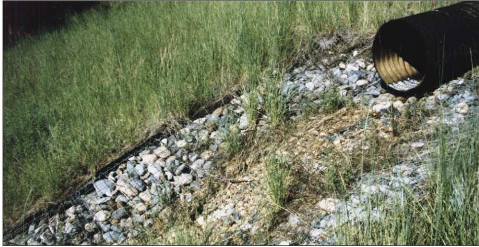
Photo 122. 24" bituminous-coated culvert collects cut-slope and roadway runoff, then discharges to gabion downdrain, 4 May 1995. Culvert extends beyond top of downdrain by 2 feet, prevents undermining, splash zone extends 6-feet downhill from culvert outlet, runoff flows into rock-filled gabions, energy is dissipated.
