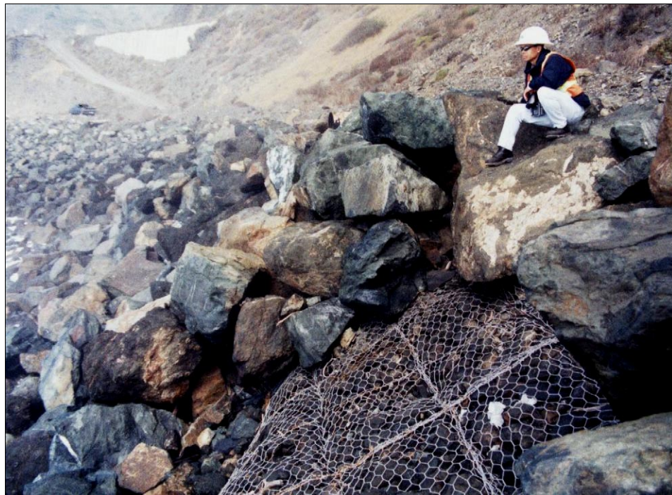
Photo 88. South RSP, looking northerly, rocks missing near top of revetment, some gabions exposed, 4 Nov 1998. Light rock displaced from lower part of revetment by above-normal waves of January 1997 storms, then rocks above the displaced lower rocks fell down slope, exposing mattresses. We saw one exposed zone among south RSP, while we saw several exposed zones among north RSP.
