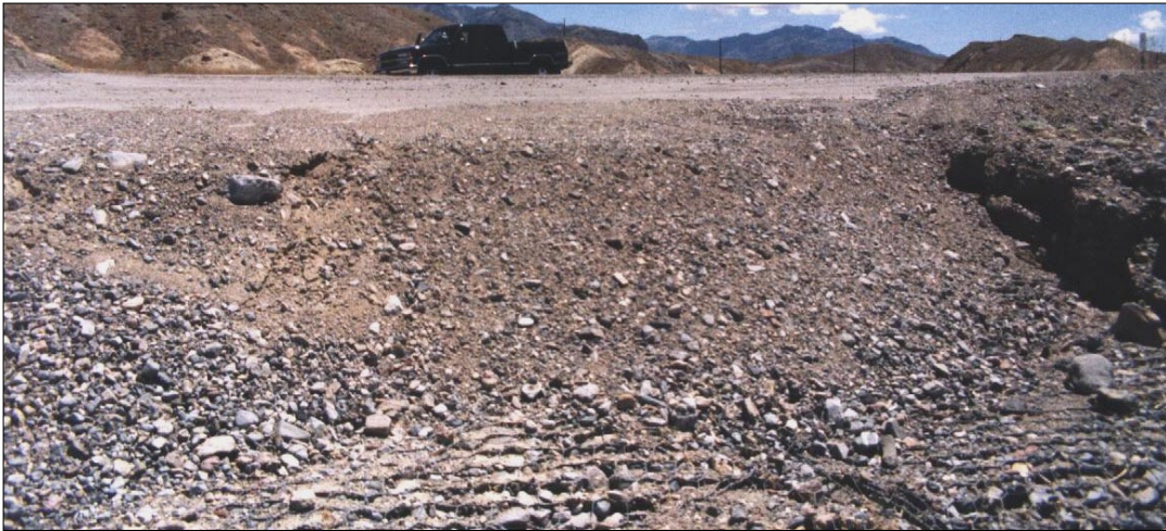
Photo 111. Flood washed-out road in 1983. Looking up-slope and upstream on 9 Jun 1998, at road fill protected by 1-foot high zinc-coated gabions, product 4. Flood waters in Gower Wash originate in mountains (distant background) and then flow across road (pick-up truck in center of channel on opposite side of road).
