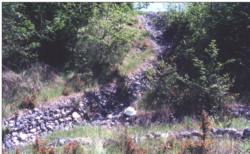
Photo 58. Looking uphill at gabion downdrain and confluence (hard hat for scale) with gabion channel (flow is to left) that gets runoff from road shoulder gully. OK after 11 wet seasons.
