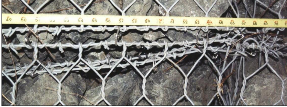
Photo 141. First of 3 out-of-specification joints using interlocking fasteners, lack of inspection and/or attention to Caltrans plans and specs. Supplier brochure showing fasteners at 6-inch intervals is not recommended by Caltrans. Caltrans requires one alternative fastener in each mesh opening along the joint, and if one fastener can not enclose all the wires in a single pass, then standard 13.5-gage tie wire must be used.
