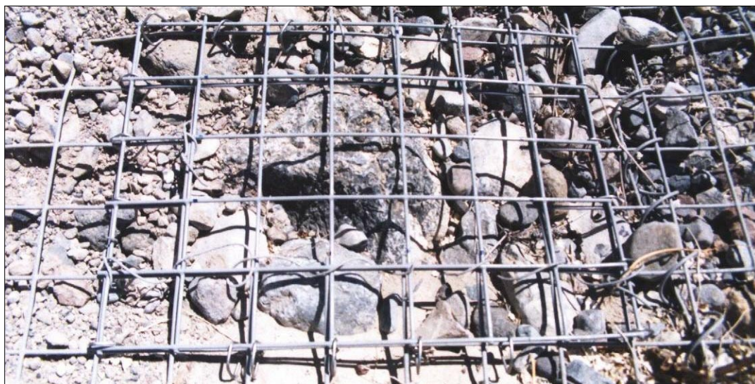
Photo 110. Completed repair. One stainless steel interlocking fastener placed in each mesh opening.
