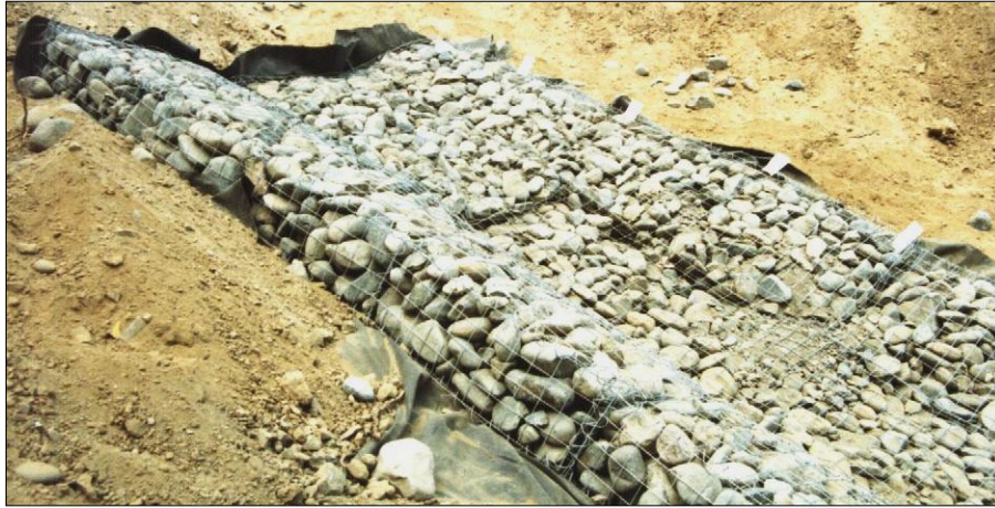
Photo 116. Building an open channel gabion downdrain, Sep 1987. First welded mesh gabion downdrain in Caltrans, made from product 1. Trapezoidal section, 1-foot high mattresses, 15H:1V side slopes, 3-foot wide bottom, woven filament geotextile underneath, 3' x 3' x 6' long counterforts every 43 feet. Longitudinal (downhill) slope is about 2H:1V. As with most culverts, installation proceeded from low to high elevation.
