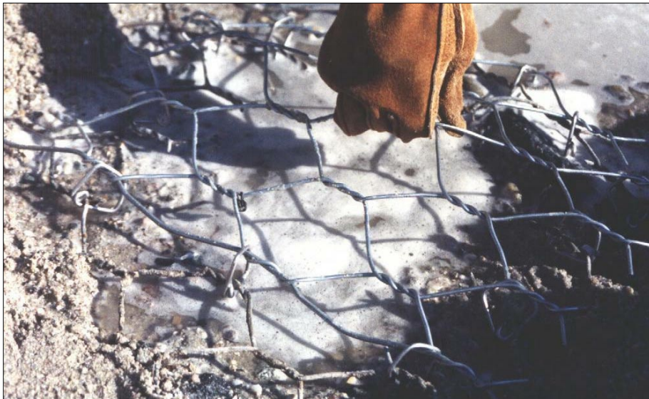
Photo 132. After collecting sample of check dam, lid panel was repaired with new section of product 4, 11-gage zinc-coated mesh and interlocking fasteners.
