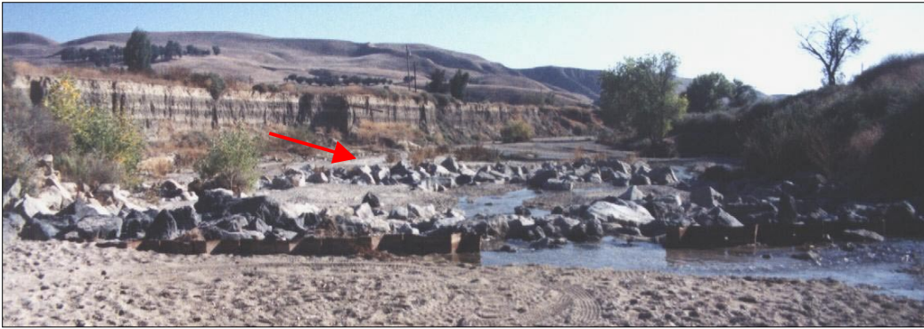
Photo 128. Looking downstream over sheet pile check dam. Piles of bridge 49-0095 were exposed, because creek bed degraded from downstream gravel mining and constricted channel. Check dams built in 1996 upstream and downstream of bridge, temporary scour countermeasures. Creek bed elevation raised 4 feet to about elevation 1024 feet. Prior 1-ton riprap around pier washed downstream (arrow).
