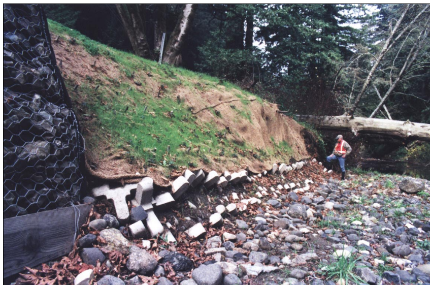
Photo 164. Abrupt change from gabion wall transitions to stream bank with 75-pound interlocking concrete armor units (AJACKS) to prevent toe erosion beyond wall.
