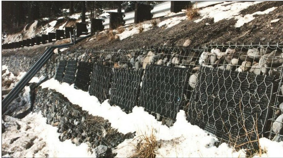
Photo 76. Gabion wall made from product 1 after 1 year, 21 Nov 1990. Test panels had mostly air exposure, except in winter they were partially covered with snow. This image is after 1 st snow near start of 2 nd wet season. Snowmelt had roadway deicing salt.
