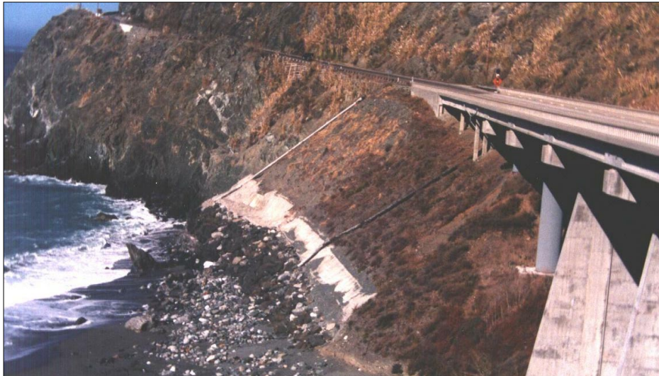
Photo 155. Walls buttressed by 8-ton rock, built 1995, looking northerly, 5 Nov 1998. Nonwoven, heavy-duty (16 oz / sqyd), high permittivity ( >0.5 per second) RSP-fabric initially placed on beach and against walls.
