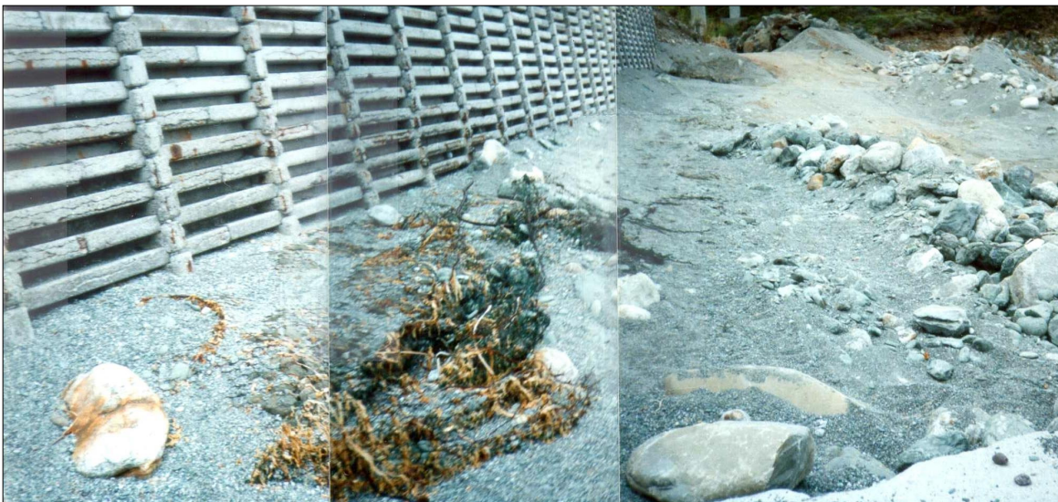
Photo 154. During 6 th wet season, waves and rocks hammered new crib wall, some gabion cells were emptied by wave action, boulders were strewn about, looking southerly 15 Aug 1995. By this time, new crib wall was so distressed, it needed to be replaced or buttressed.
