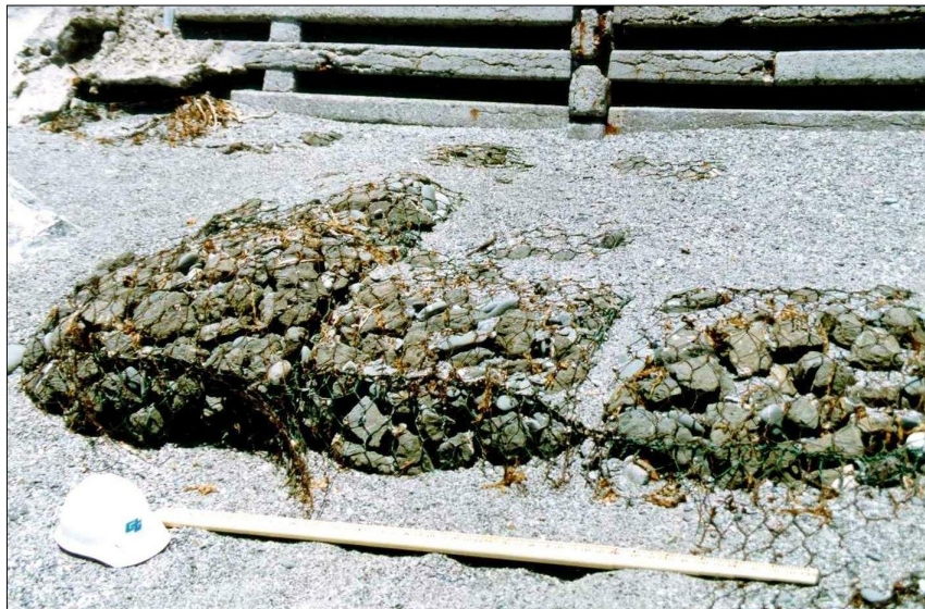
Photo 153. After 5 wet seasons, near join to old crib wall, gabions on left OK, while gabion at right failed, part of lid was opened, right foreground, 1994.
