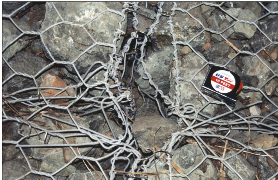
Photo 143. Third of 3 out-of-specification joints, four baskets not joined at corners, where multiple basket-to-basket joint is required. It appears empty baskets were laid out and filled with rock, then rocks were crammed into void where tied joint should be. Such practice is contrary to Caltrans and most supplier specifications, which require : form single baskets, join them, slightly over fill them with rock, close and fasten the lids.
