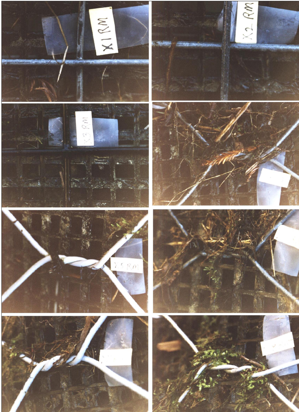
Photo 3. Close-ups of gabion test panel wires. Done for most site inspections. Number of inspections ranged from as few as 1 to as many as 7 visits in about 10 years. From left to right and from top to bottom, images are respectively gabion mesh wires of :
