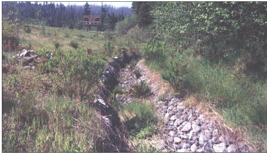
Photo 54. downdrain OK after 11 wet seasons, 26 May 1999.
