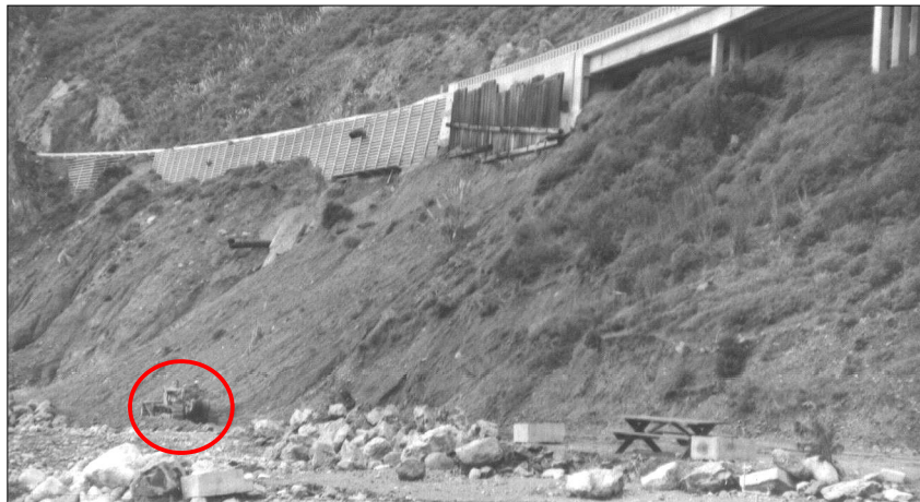
Photo 146. On 7 Jan 1974 slope failed below abutment 10 and approach road crib walls. Looking northerly from beach. On 9 Jan 1974 dozer (circle) started grading for near sea-level crib wall to stabilize toe. Continual toe erosion, twice daily high tide to elevation 6 feet, storm waves seen higher than elevation 25 feet.
