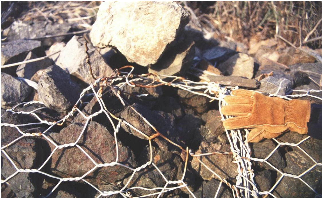
Photo 97. Corners and tread (horizontal portion) of stepped walls are intermittently impacted by rocks. Rocks slough from slopes above walls. Pacific Coast Highway is about elevation 60 feet. Top of wall is about elevation 25 feet, approximate reach of storm waves.
