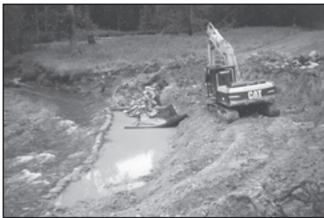
Figure 9. July 1999. Using sandbags and trash pump to control sediment during construction of revetment at Site F.
