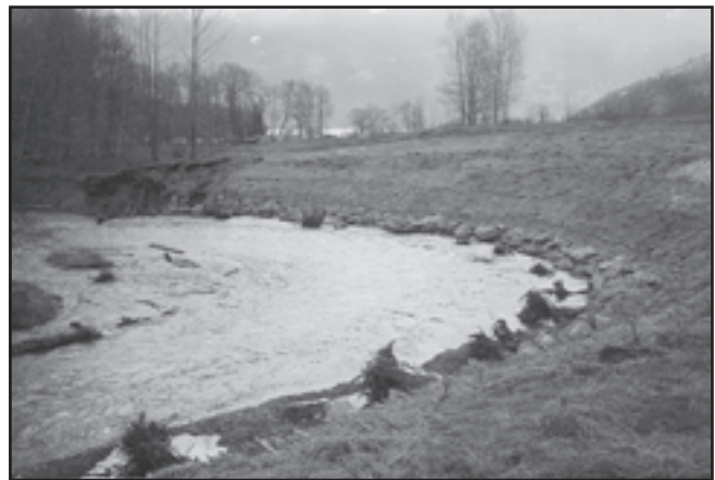
Figure 4. April 1999. Site B during freshet immediately following construction. Note low velocity areas created by rootwads.
