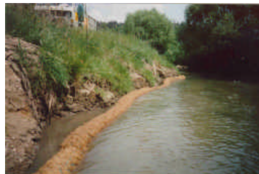
Figure 2. CGR on German stream 1 year after installation (photo courtesy of Bestmann GmbH, Wedel, Germany)
