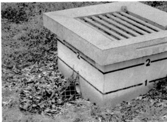
Functional trash rack
