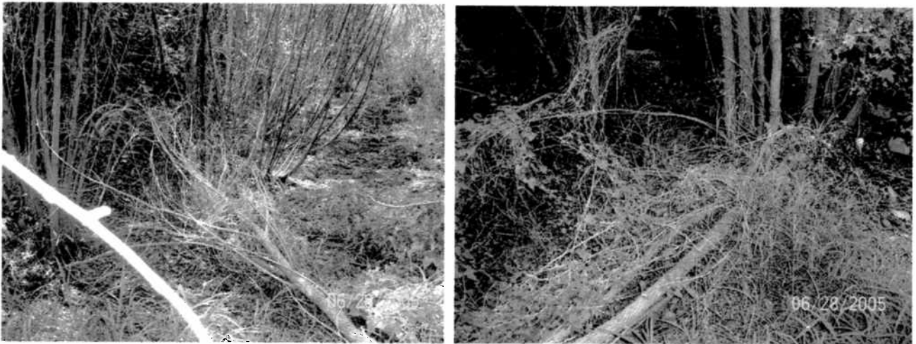
Fallen and dead woody vegetation can cause blockage in basin and possibly block outlet
