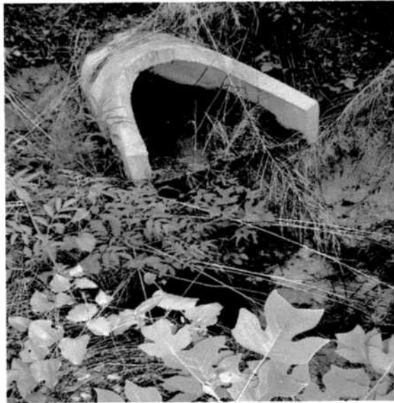
Outlet at downstream embankment w/major erosion
