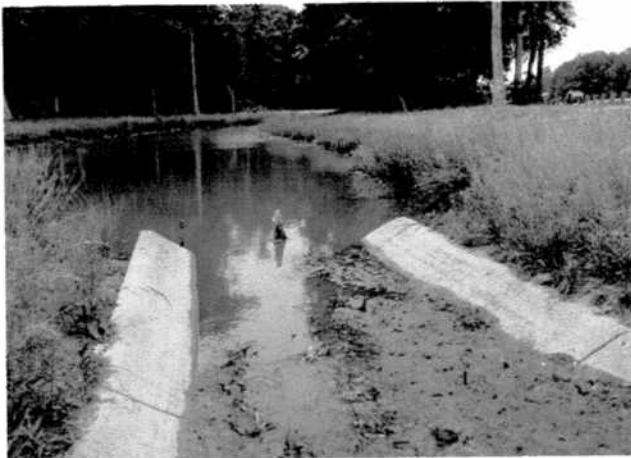
Major "Ponding" due to blockage of outlet
