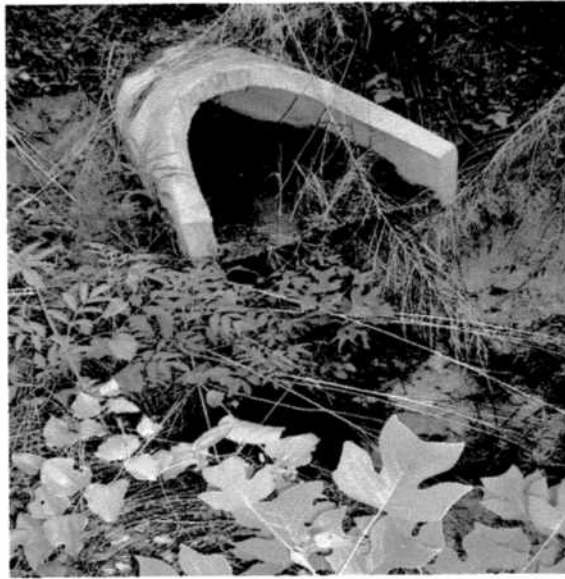
Outlet at downstream embankment w/major erosion
