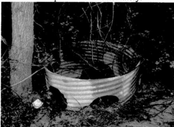
Riser chamber w/excessive amount of sediment
