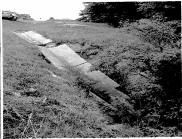
Un-stabilized conveyance channel into Basin inlet
