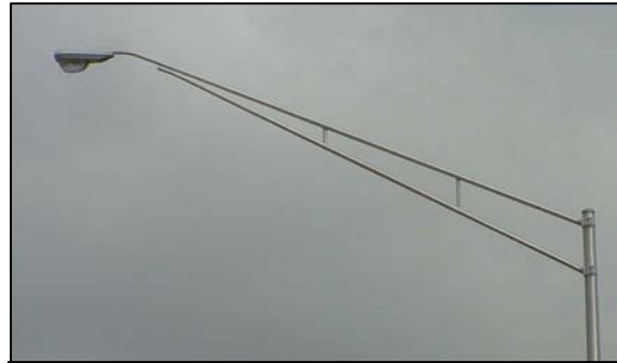
Figure 2-11: Luminaire Bracket Arm
