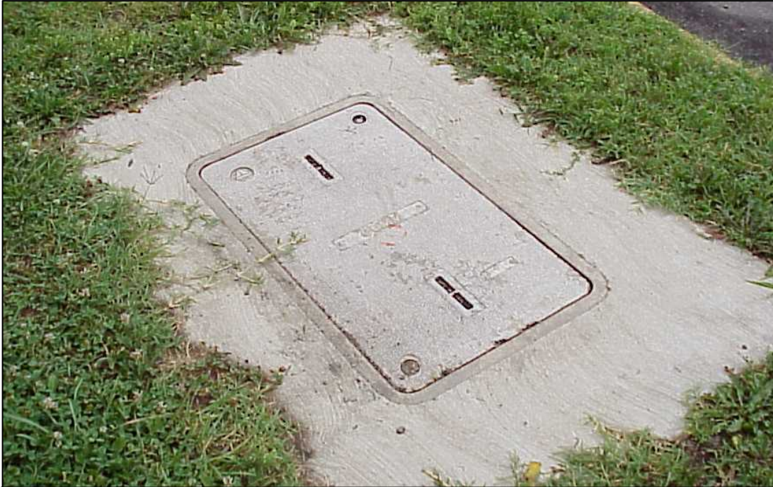
Figure 2-19: Standard VDOT Junction Box
