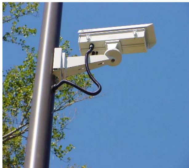
Figure 2-9: CCTV Mounted to Light Pole
