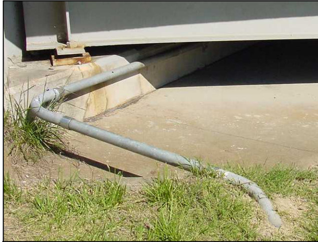
Figure 2-20: Exposed Metal Conduit
