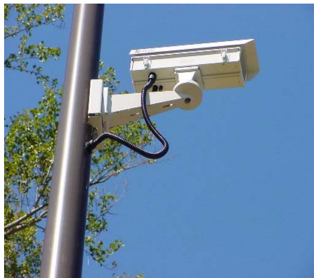
Figure 2-9: CCTV Mounted to Light Pole
