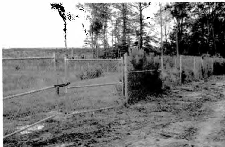
Fence surrounding Basin with gate unsecured and saplings growing in fence line
