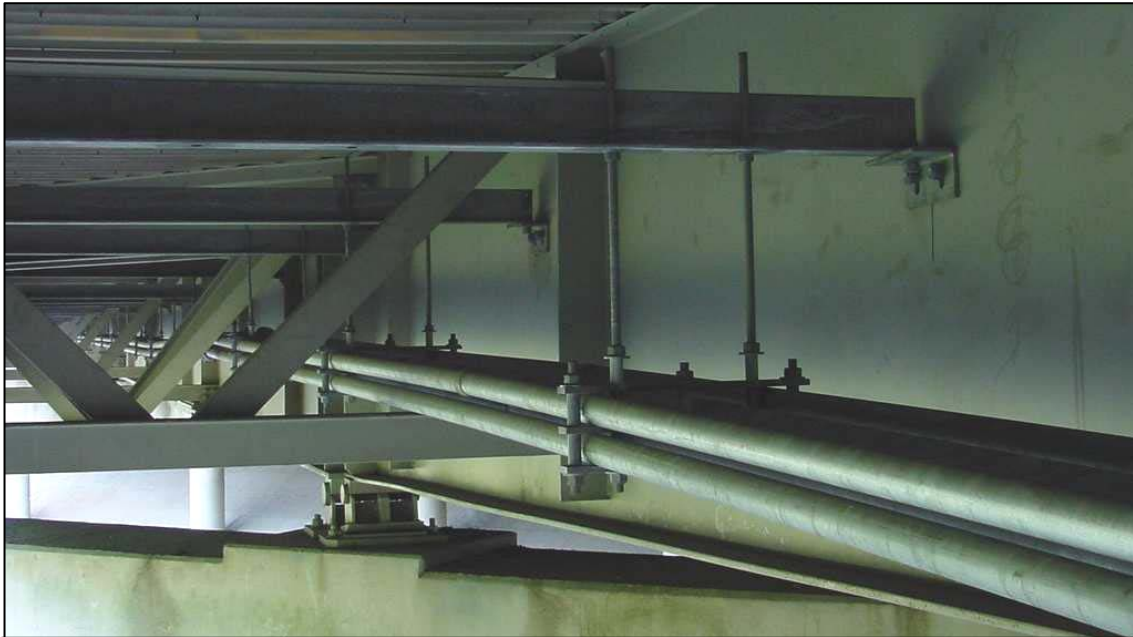
Figure 2-21: Under Bridge Conduit Support System
