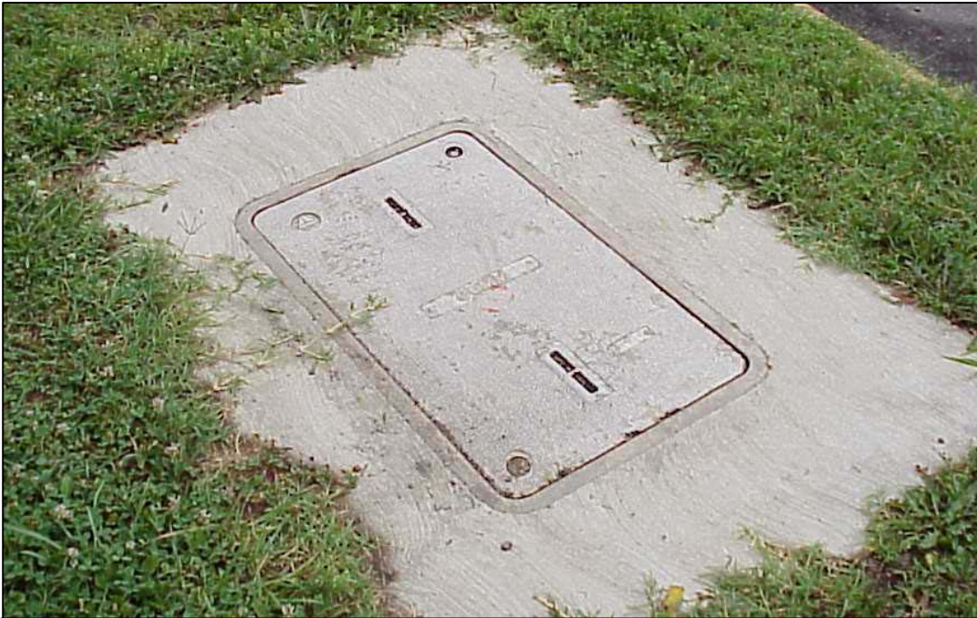
Figure 2-19: Standard VDOT Junction Box
