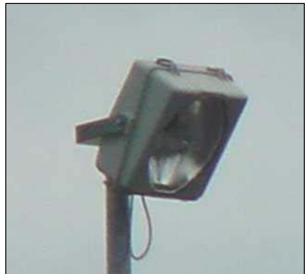
Figure 2-9: Offset Luminaire Note: VDOT lighting designs no longer use non-cutoff tilted luminaires.
