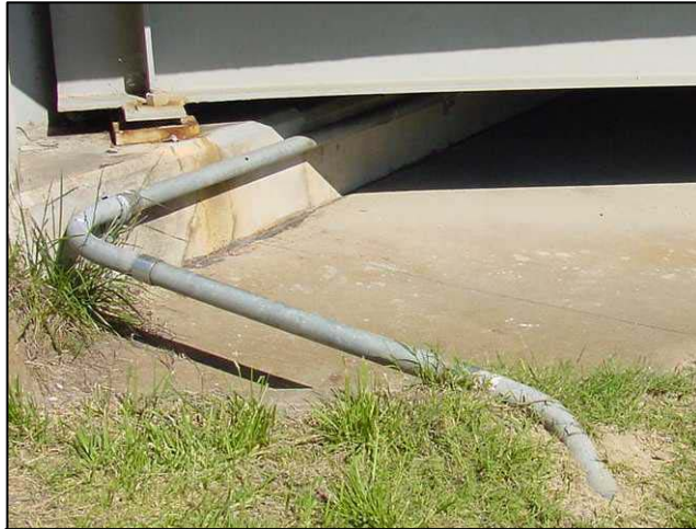
Figure 2-20: Exposed Metal Conduit
