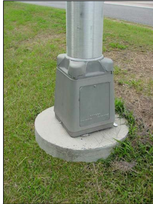
Figure 2-15: Transformer Base on LF-1 Foundation.
