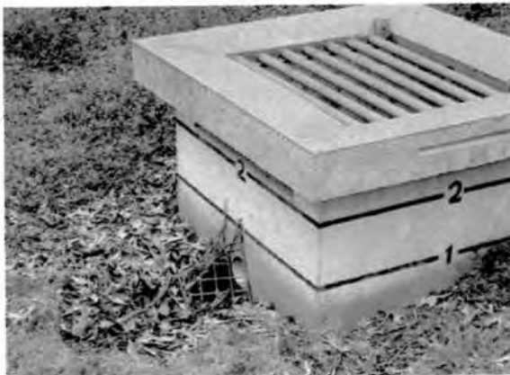
Functional trash rack
