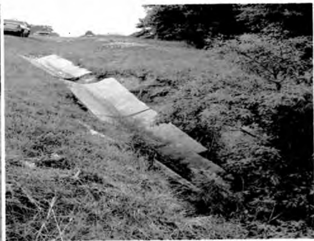
Un-stabilized conveyance channel into Basin inlet
