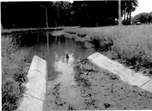
Major "Ponding" due to blockage of outlet
