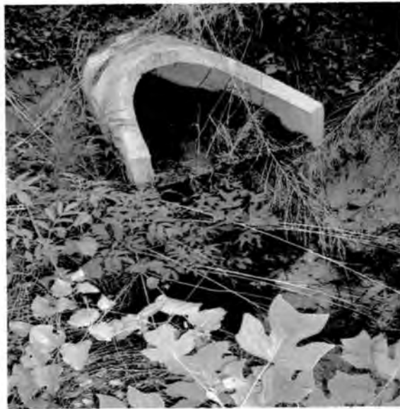
Outlet at downstream embankment w/major erosion
