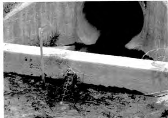
Trash Rack blocked by silt/mud and plastic
