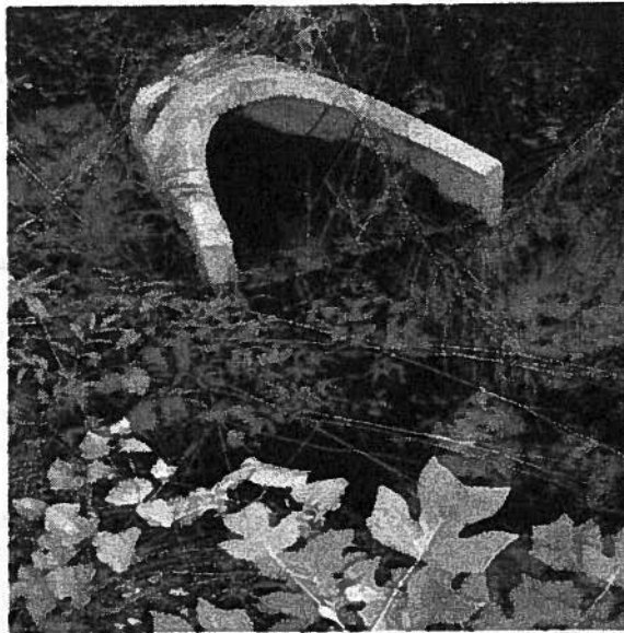
Outlet at downstream embankment w/major erosion
