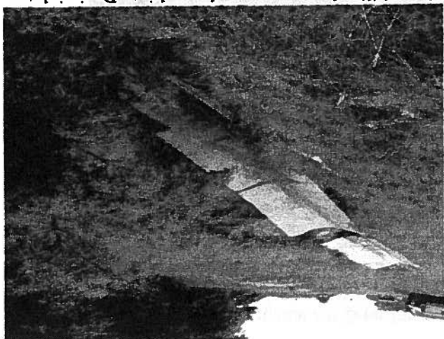
Un-stabilized conveyance channel into Basin inlet
