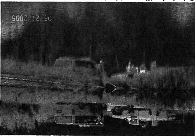
Principal spillway with pipe only, no structure
