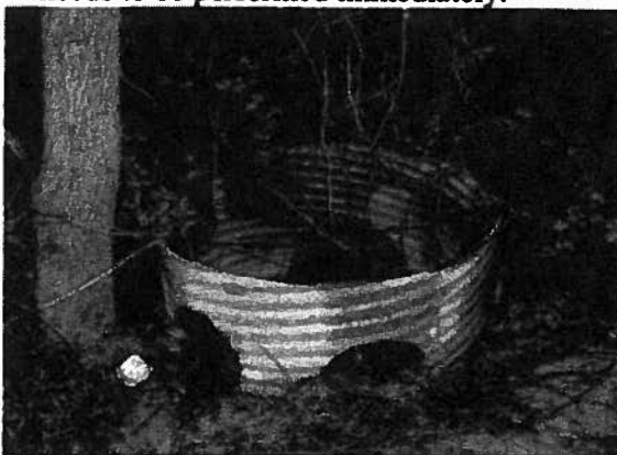
Riser chamber w/excessive amount of sediment
