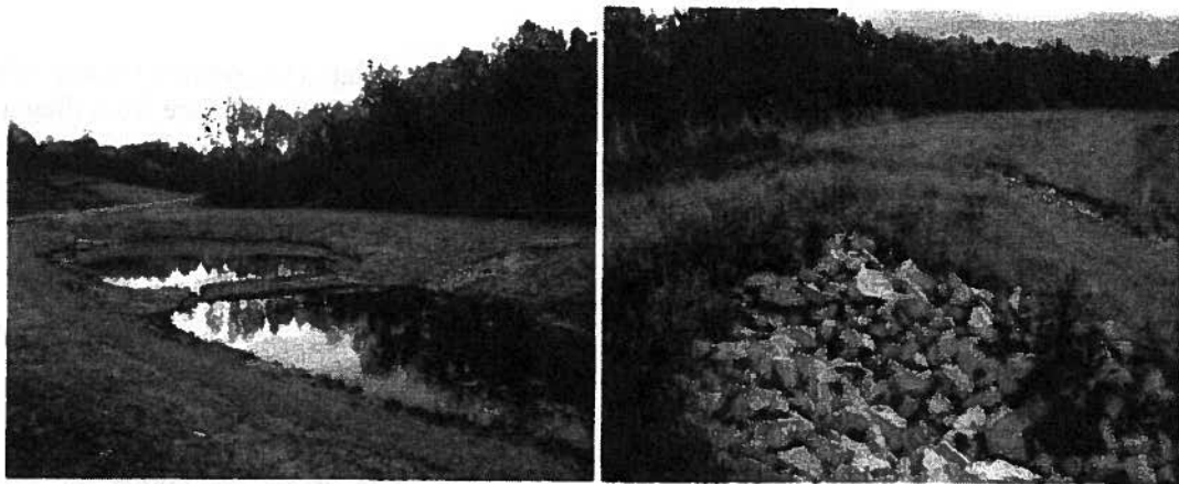
Good access to Basins as well as all the way around Basins for maintenance
