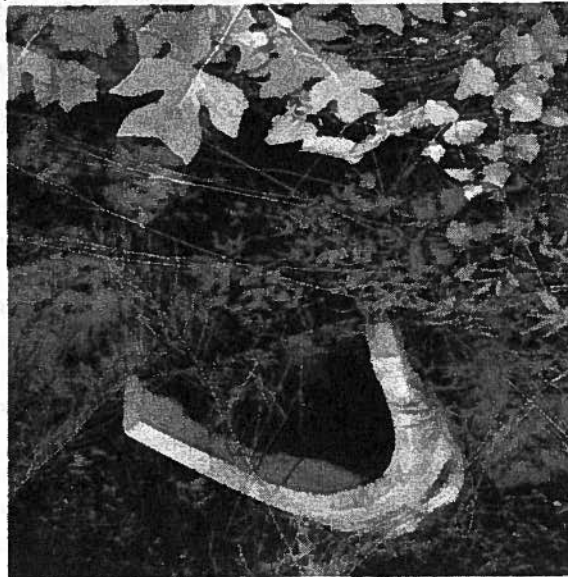
Outlet at downstream embankment w/major erosion
