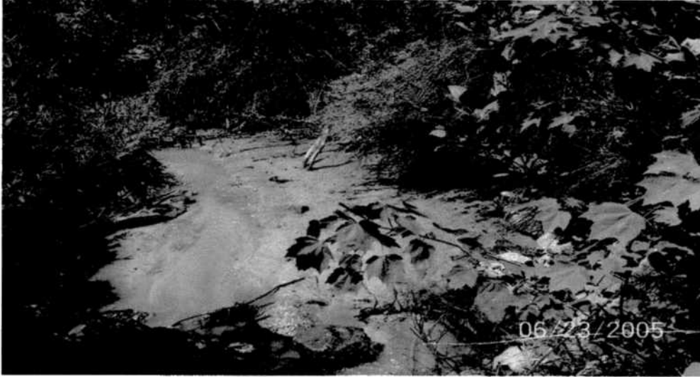
Sediment build-up in inlet due to conveyance channel instability
