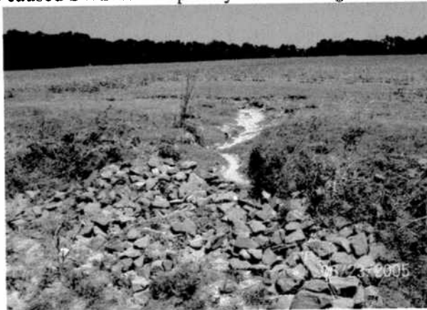
Erosion in watershed upstream of Basin inlet
