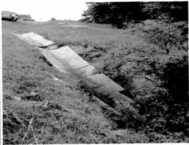
Un-stabilized conveyance channel into Basin inlet
