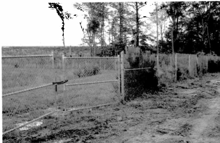
Fence surrounding Basin with gate unsecured and saplings growing in fence line
