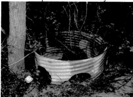
Riser chamber w/excessive amount of sediment
